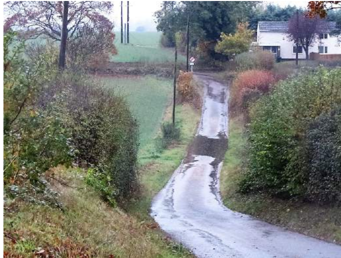
Photograph 20: Old Lane Vertical Alignment with Standing Water
