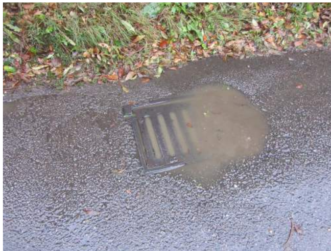
Photograph 6: A Blocked Gully on Swangleys Lane
